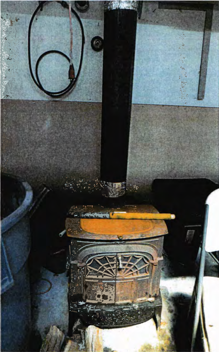
Maintenance garage – furnace (wood burning)
