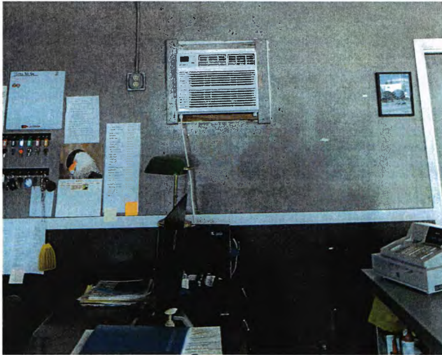
The office – wall installed AC unit
