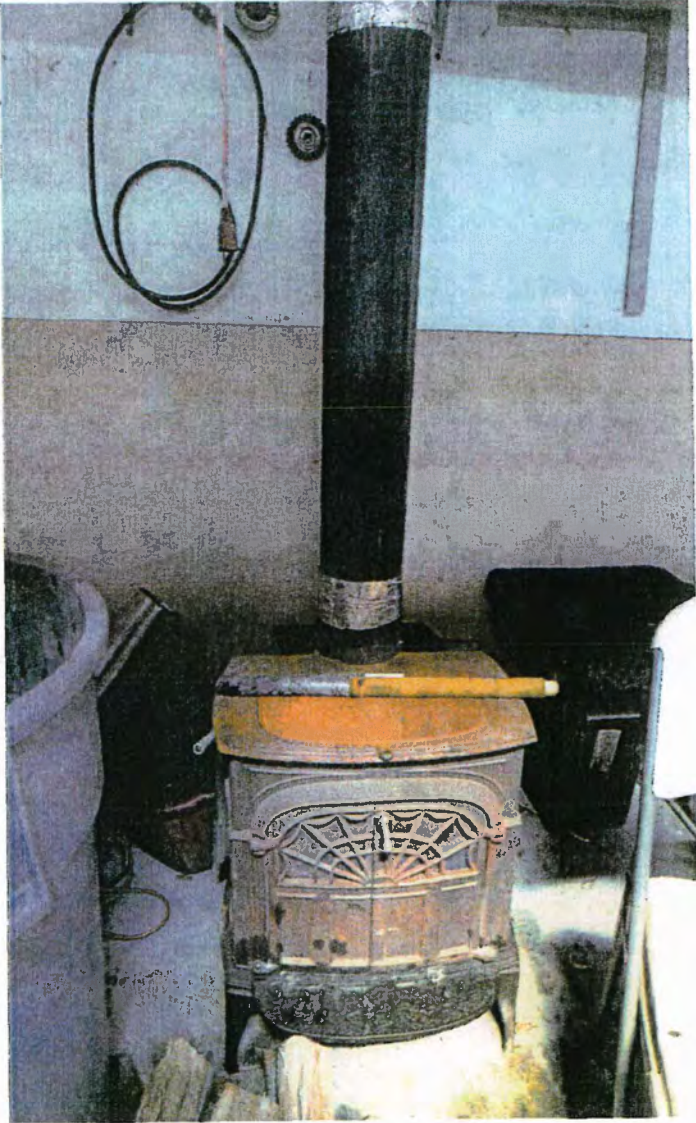
Maintenance garage – furnace (wood burning)
