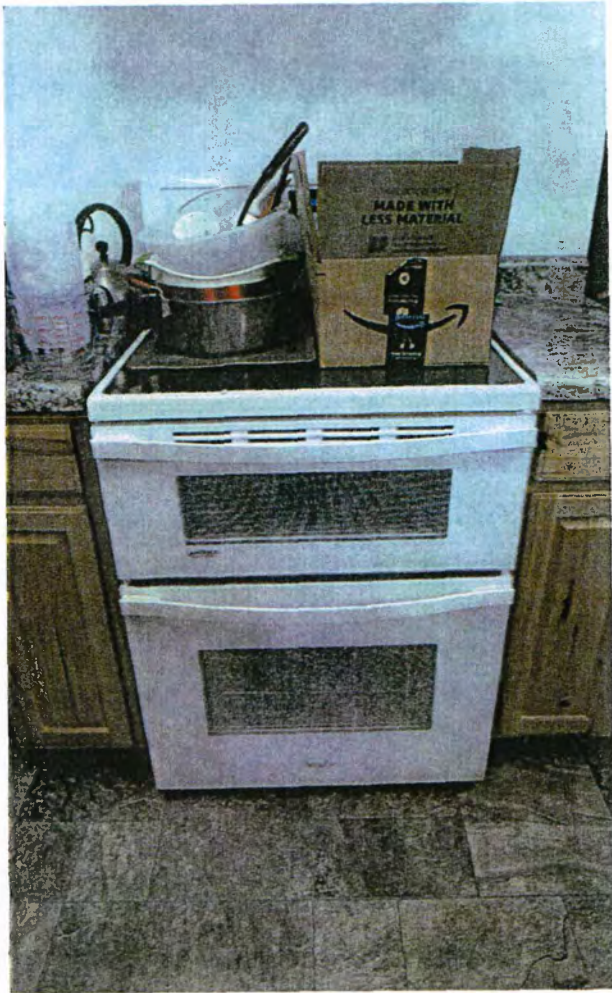
Lodge – Board Room – Whirlpool Stove
